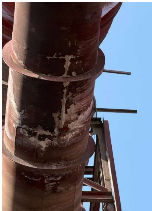
58-rasm. Gazoxod trubasining vertikal qismi – korroziyaga uchragan sirt holati
