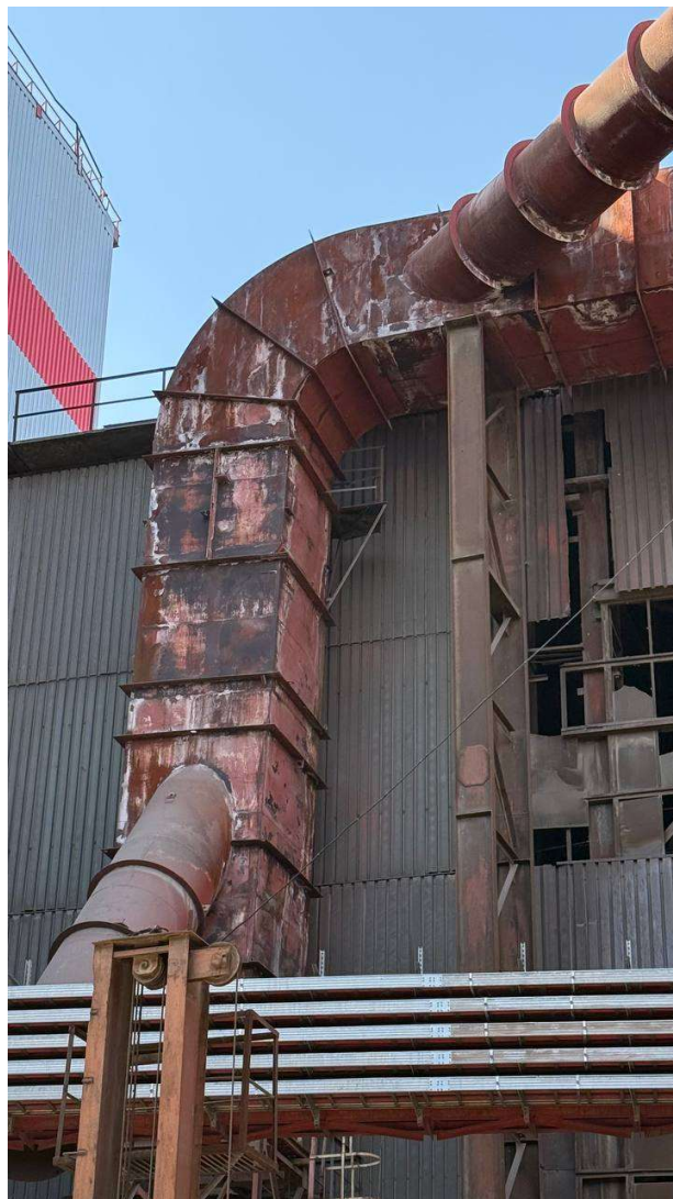
59-rasm. Gazoxodning vertikal egilma qismi – tashqi sirt holati
